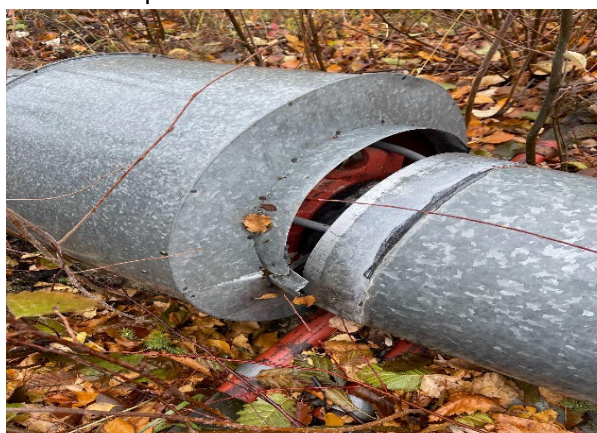
Damaged raw water transmission line
