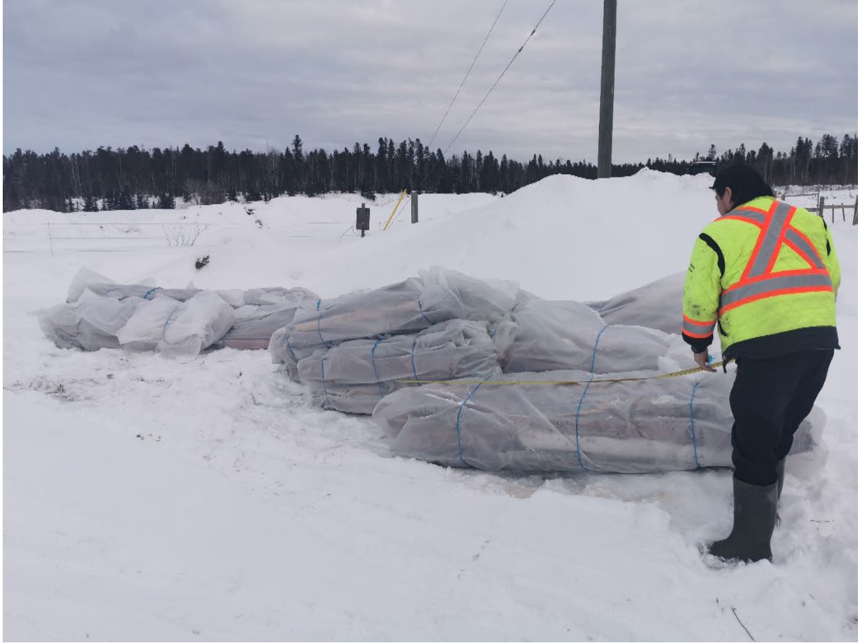
Siding from the old firehall containing lead paint wrapped and ready for transport to hazardous waste facility.
